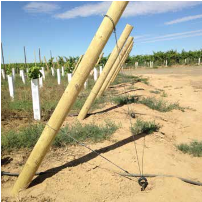
Installed in a loop format with choke knot on a wooden post
